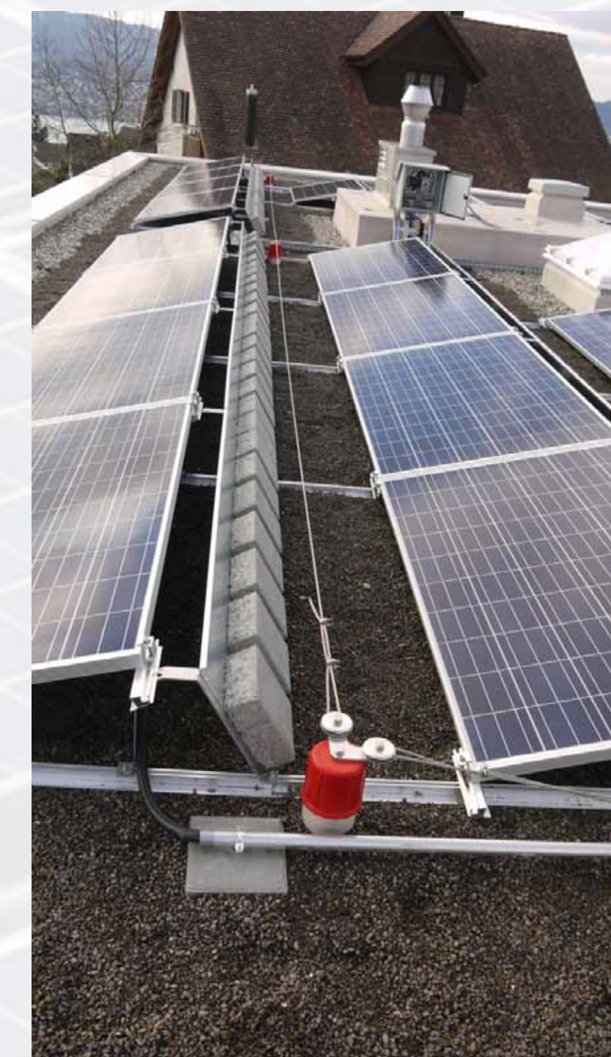
The national insurance company SUVA published requirements for safety installations necessary on buildings when operating PV plants. Costs of these safety installations can reach up to 32% of PV system costs for a 30 kW p PV plant. Avoiding installation of lifelines is only possible by accepting reduced available roof area.
