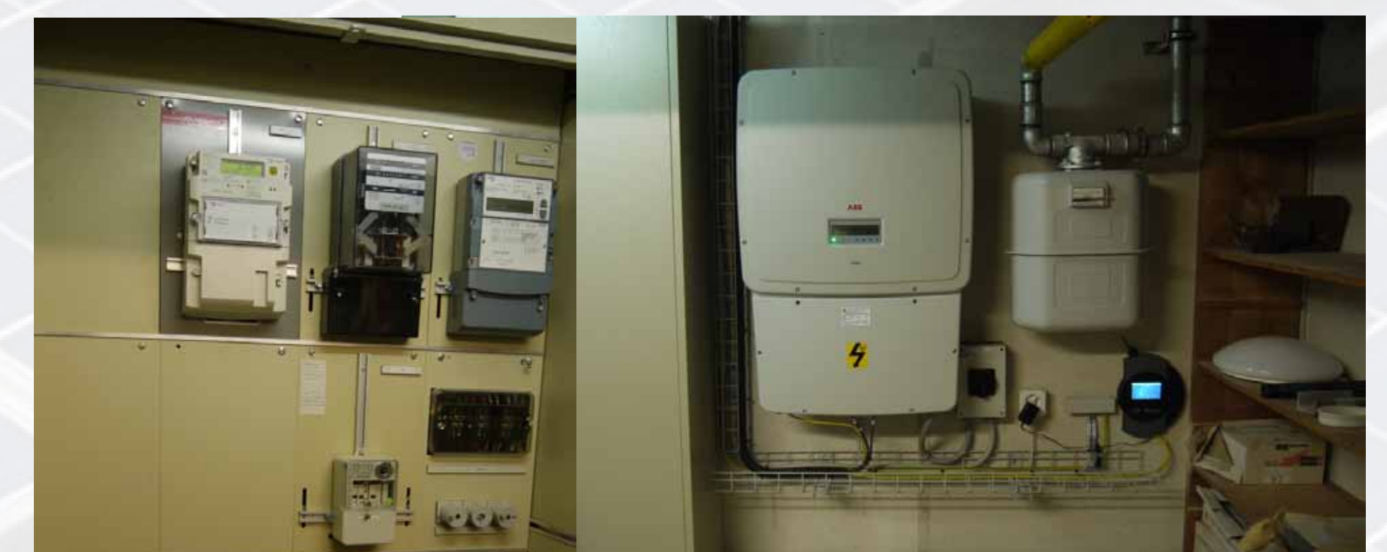
Requirements for electrical installations range from different levels of surge protection devices to firefighter switches. Different authorities publish requirements from their point of view. For PV plants with AC nominal power >30kVA, additionally special energy meters have to be installed, which have high operational costs.
