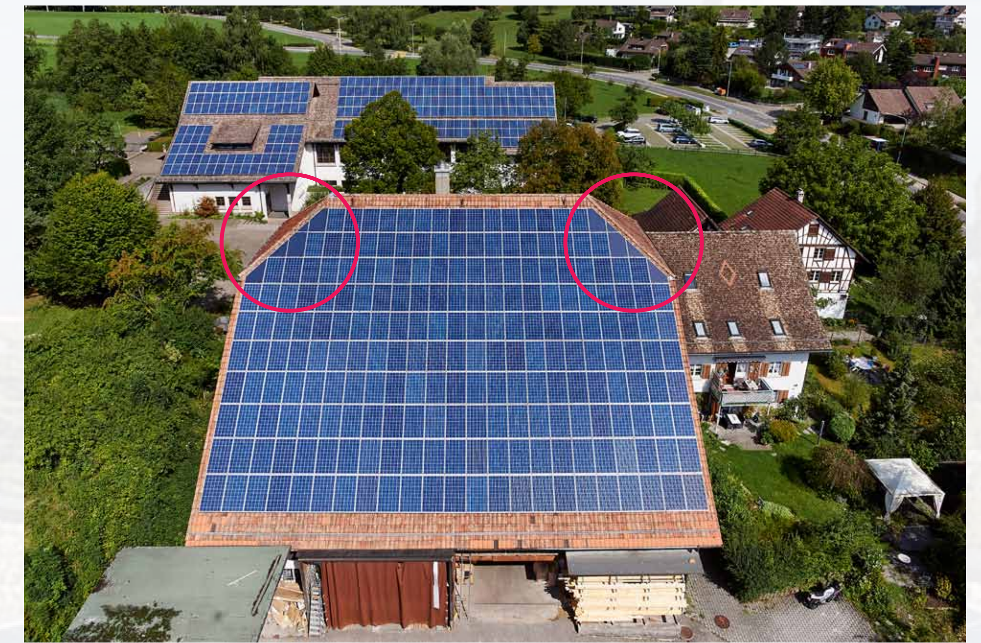
To reach a satisfactory level of integration of the PV plant and obtain the construction permit, using blind modules in corner areas of the roof was necessary.
