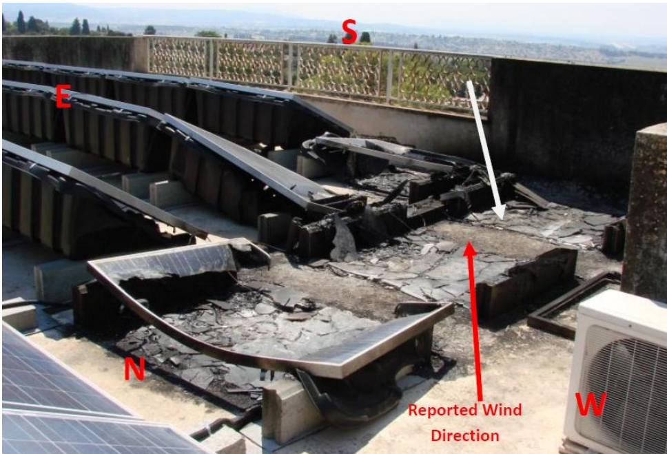
Figure 34: Fire due to junction box connection problems.
